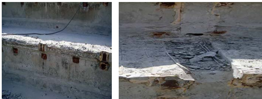
Fig. 1. Reinforced concrete construction damages of folding panels after cutting off encrustation from concrete repair mortars
